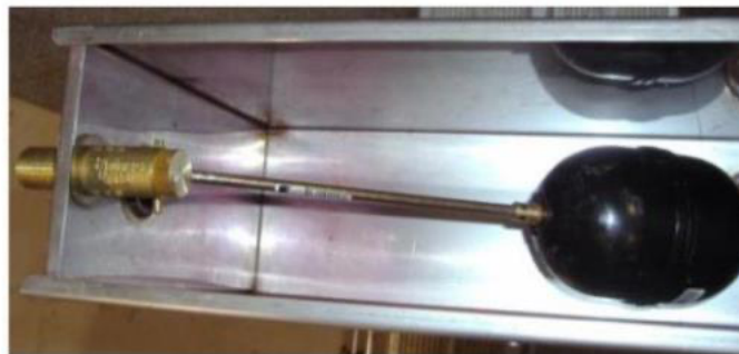
Top-up tank view from above
